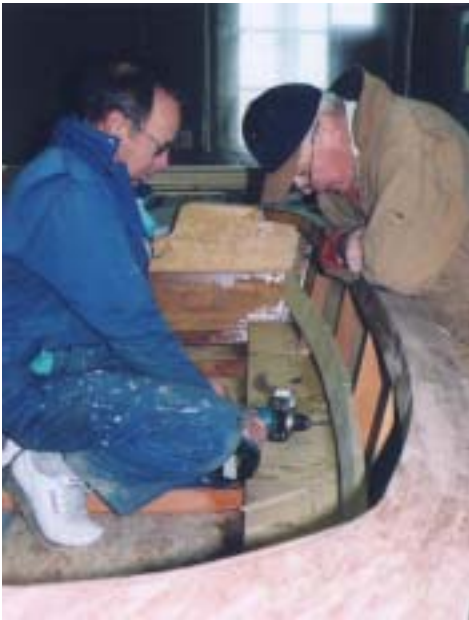
Ken Guelta and Herm Kramer work on strengthening the framework of the skiff begun by Bill Friis.
